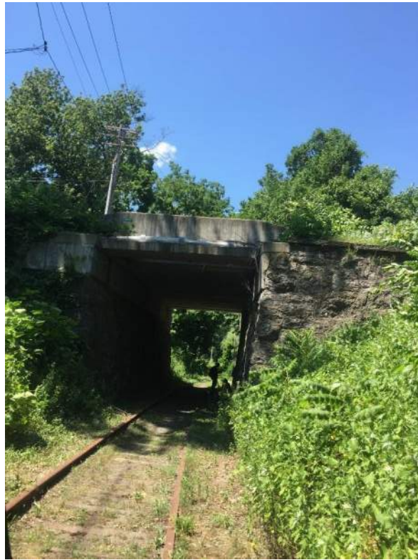
Photo 8- This photo was taken on the abandoned rail bed under Albany Avenue.
