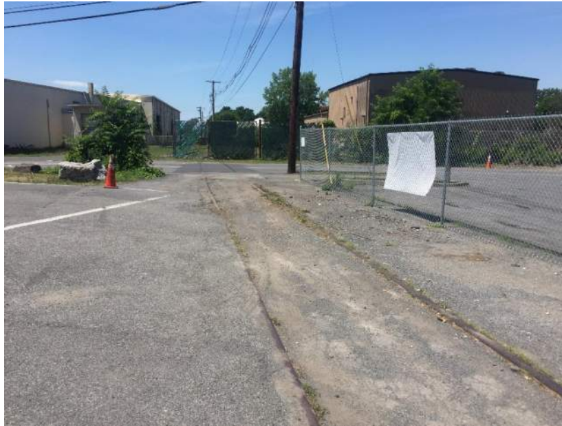
Photo 1- This photo was taken at the start of the project, where the abandoned rail bed intersects with Cornell Street.
