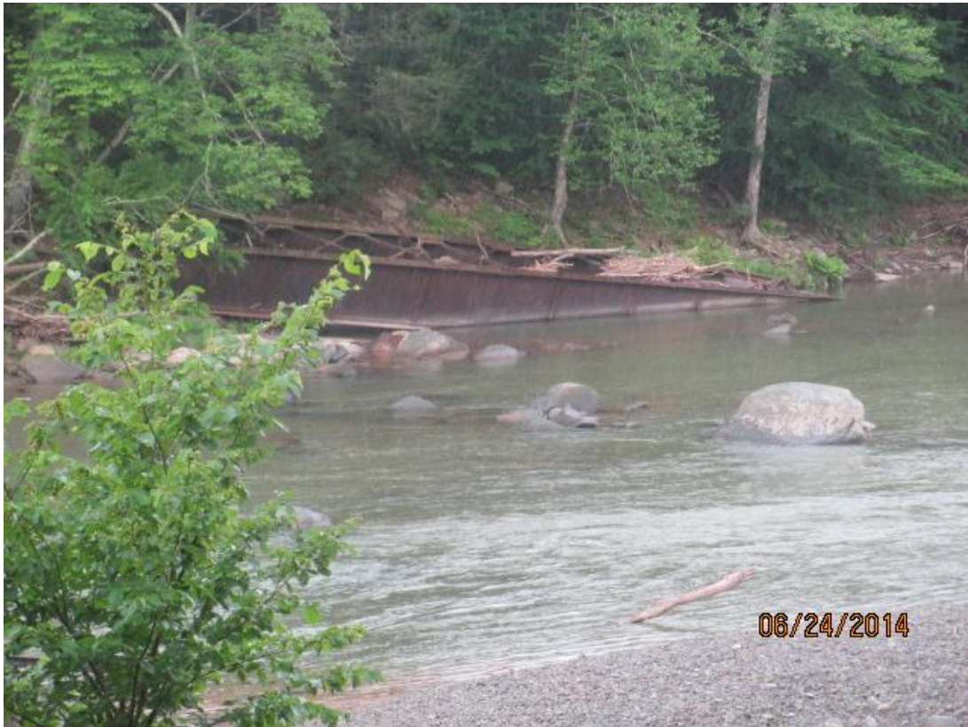
Photo 505 – Section of trestle washed up on shore
