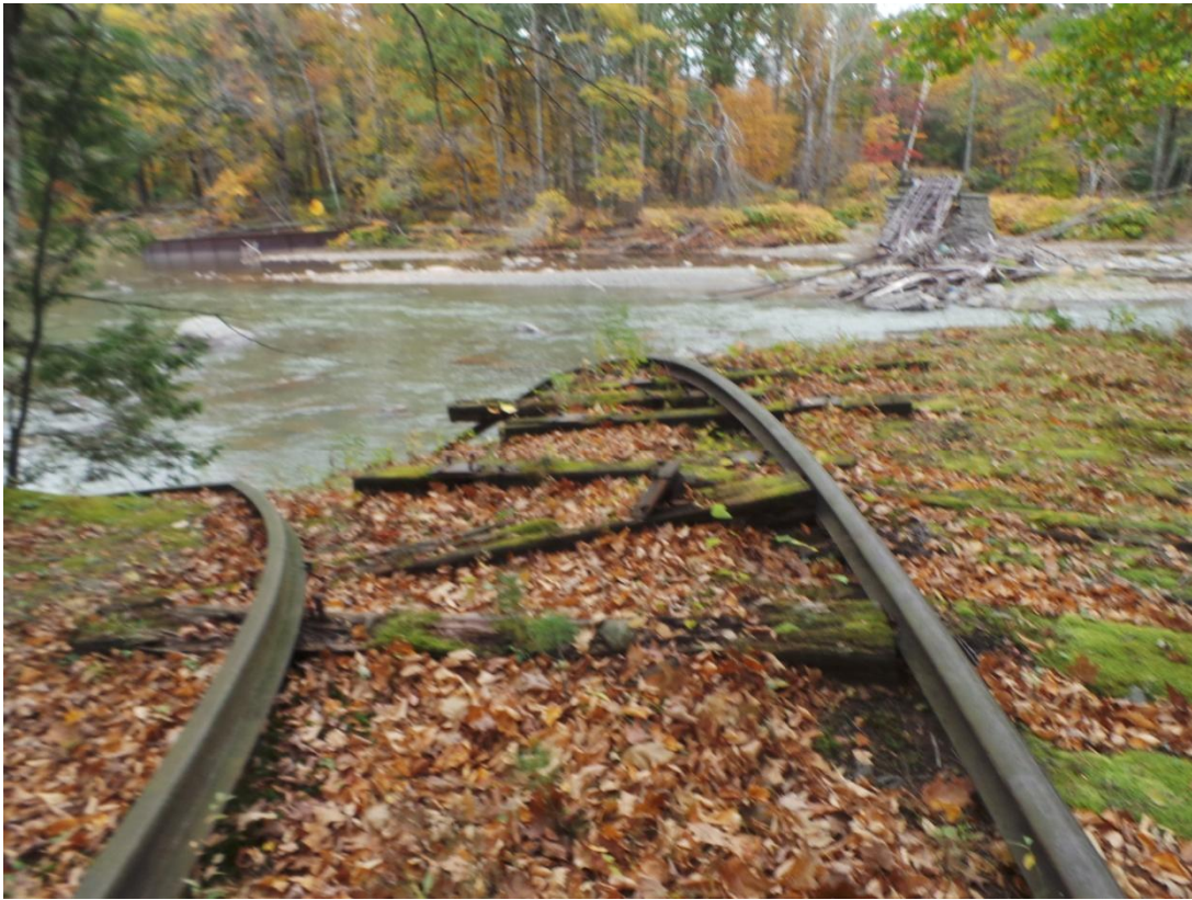
Photo 501 – Bent steel rails caused by the washout
