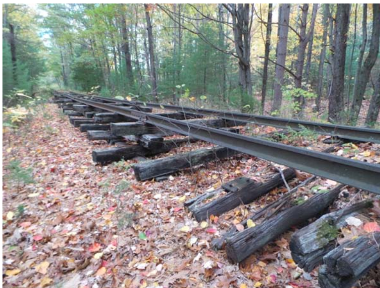
Photo 3-4 – “Cribbing” of the rails
