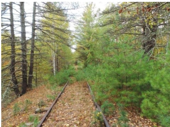
Photo 1-3 – Minor Tree Growth
