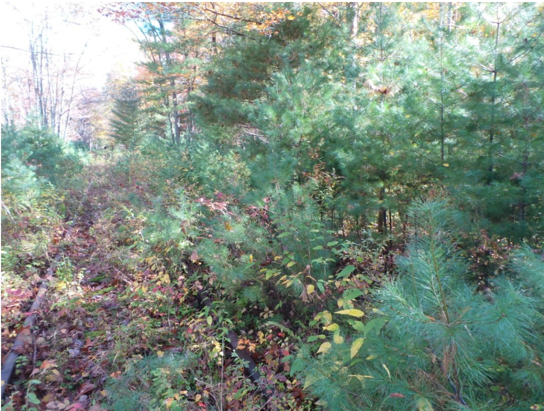
Photo 210 – Pine tree growth on rail bed and embankment
