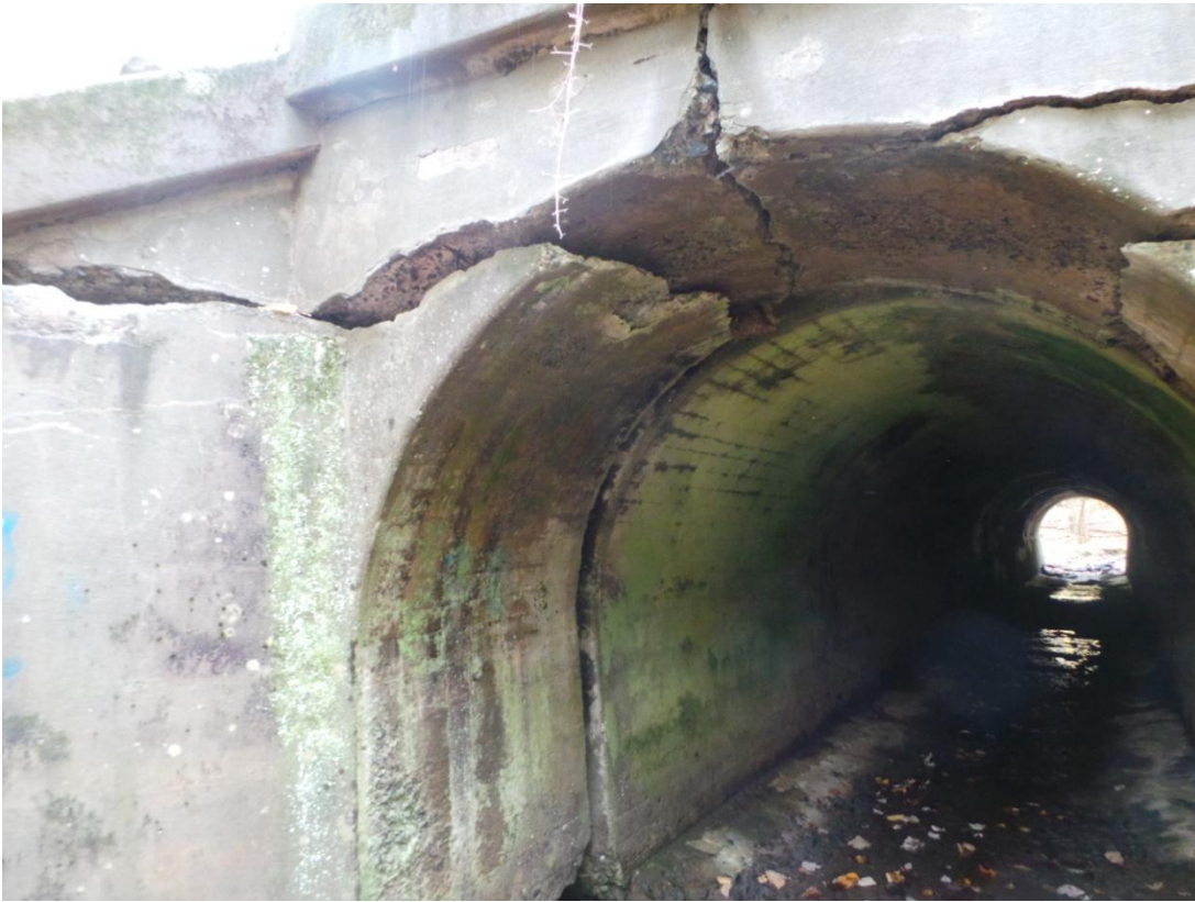
Photo 123 – Large culvert requiring wingwall repair
