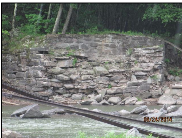
South Abutment – Dislodged Stones
