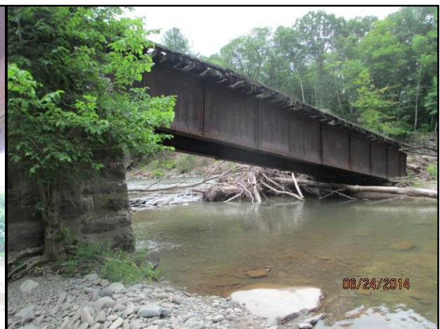
Span 2 - Dislodged From Pier 2
