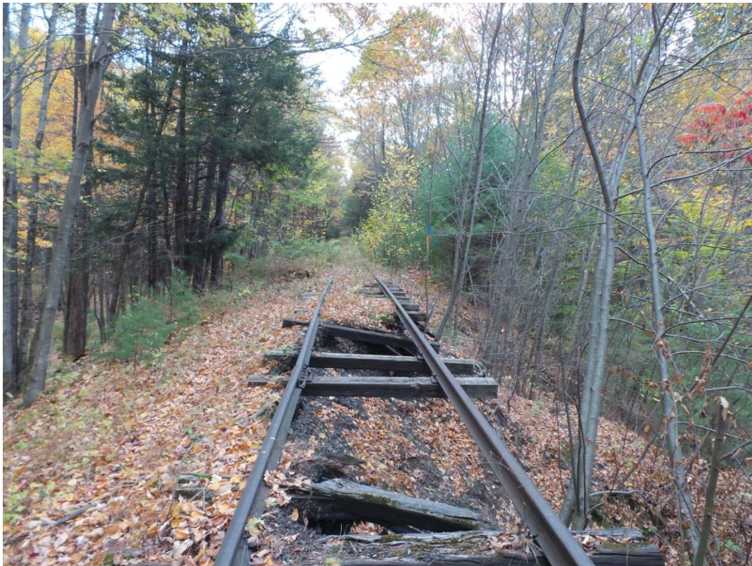
Photo 308 – Butternut Creek embankment washout
