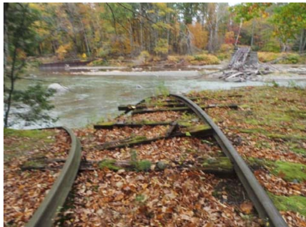
Photo 5-2 – In the background, remnants of the Boiceville Railroad Trestle over the Esopus Creek
