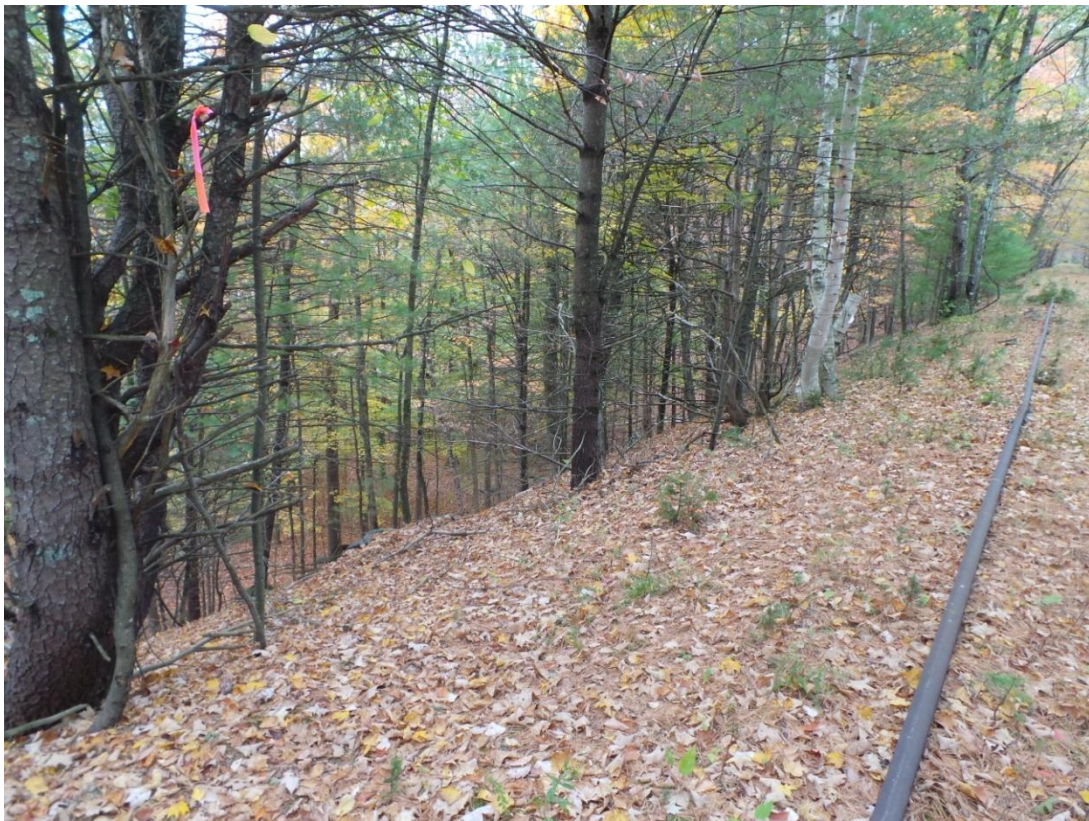
Photo 118 – Steep Fill Slope
