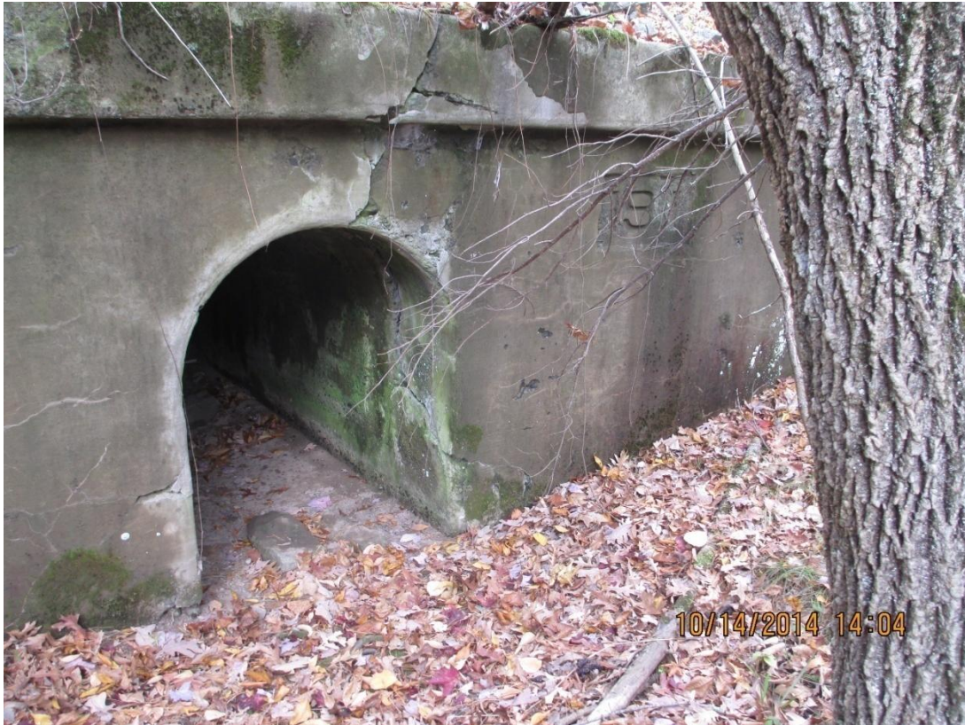
Photo 109 – Damaged culvert headwall
