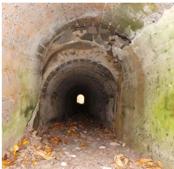
Photo 1-6 Separation and Structural Damage Inside Culvert RR Tracks Directly above Damaged Section
