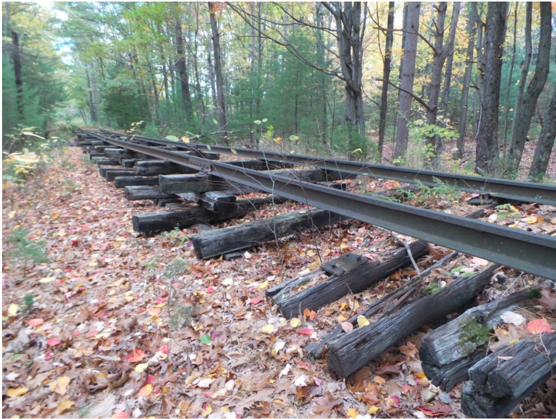
Photo 313 – Raised tracks/ballast washout
