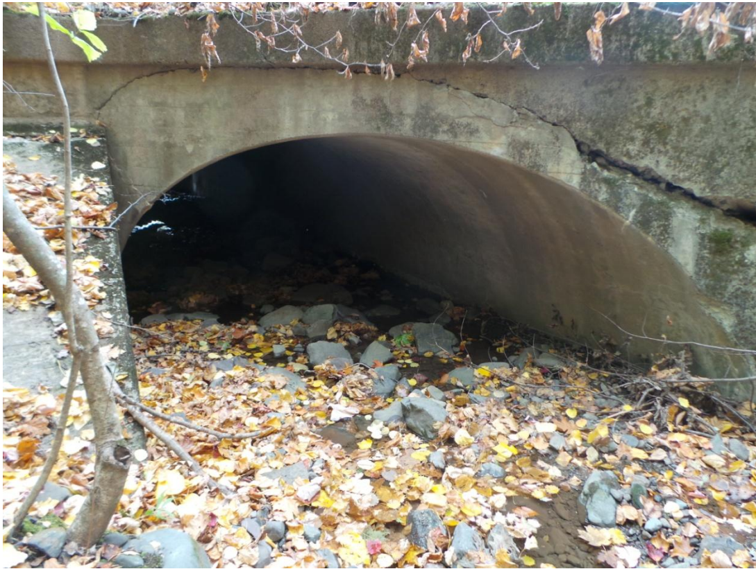
Photo 419 – Concrete culvert approximately 50% or greater filled with sediment
