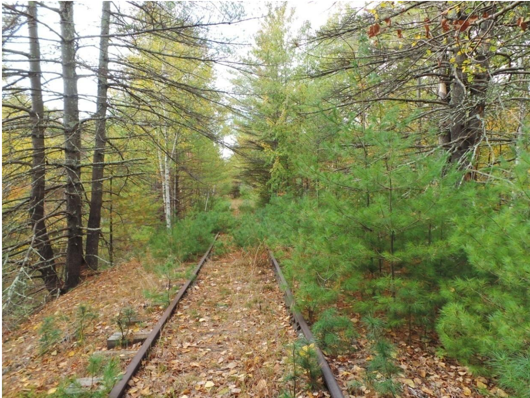
Photo 103 – minor pine tree growth on rail bed and embankment
