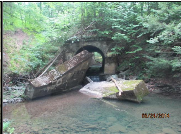
Downstream Wingwall Failure
