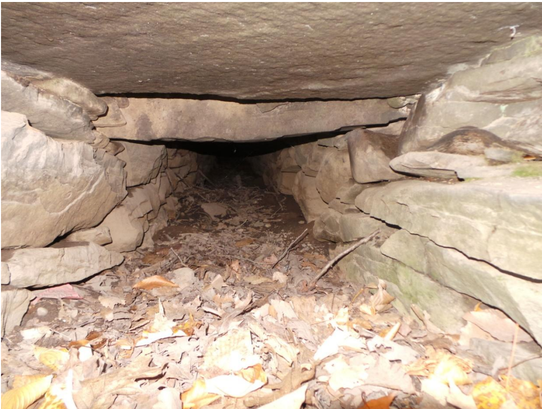
Photo 508 – Non-functional stone drainage structure
