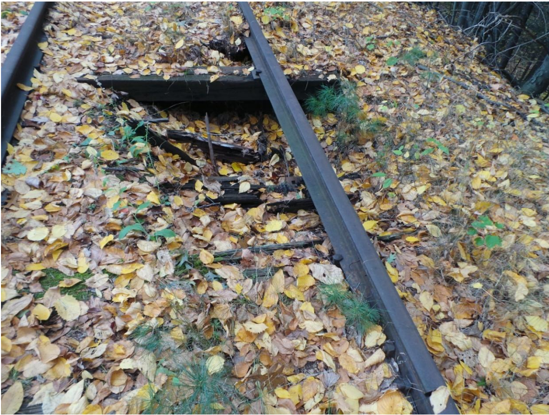
Photo 211 – Minor ballast erosion
