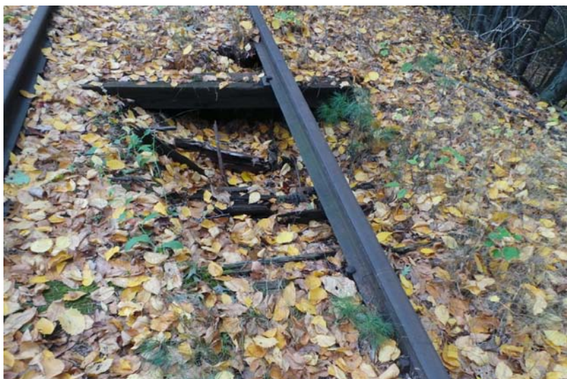
Photo 2-1 Ballast Loss and Severely Rotted Ties
