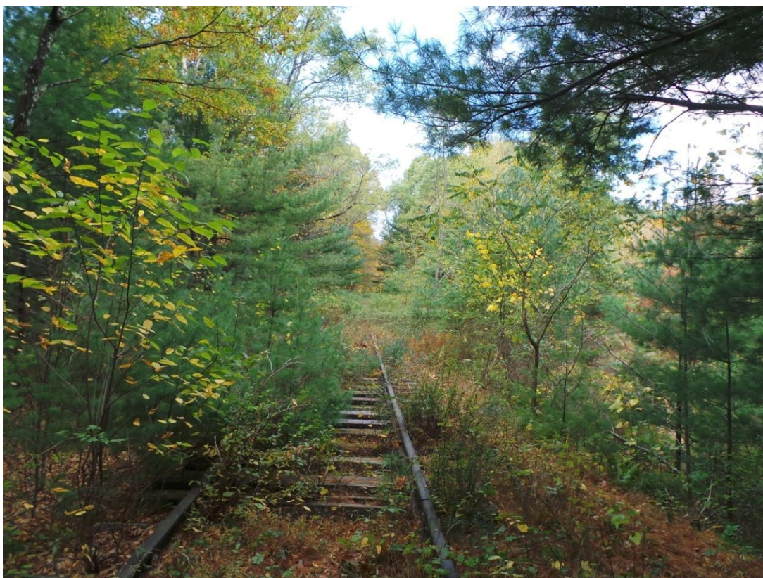
Photo 404 – Minor tree growth on rail bed and embankments
