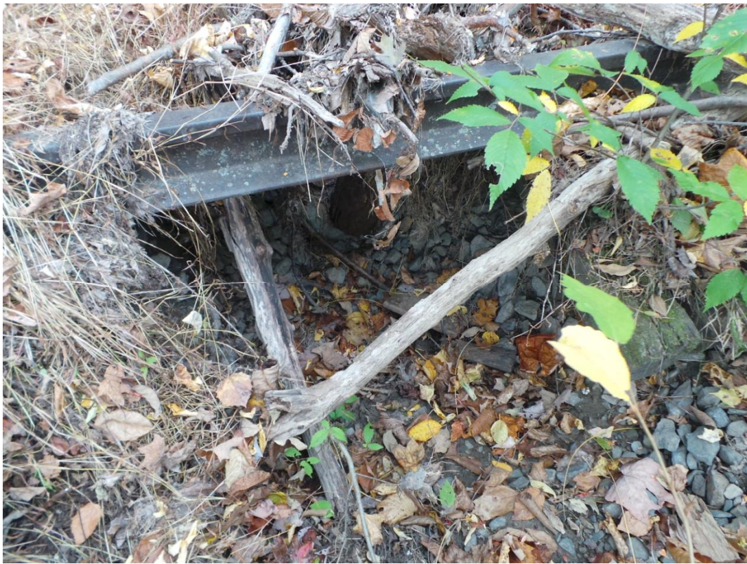
Photo 423 – Erosion of stone ballast and embankment below tracks
