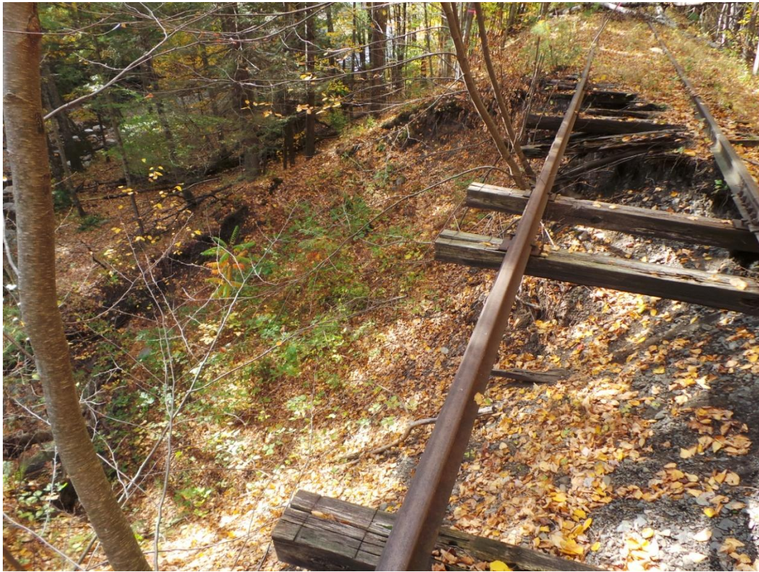
Photo 309 – Butternut Creek embankment washout
