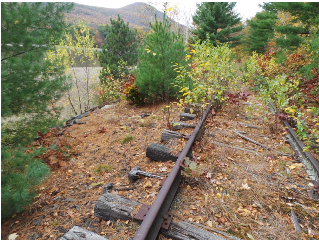
Photo 402 – Split and deteriorated wooden ties
