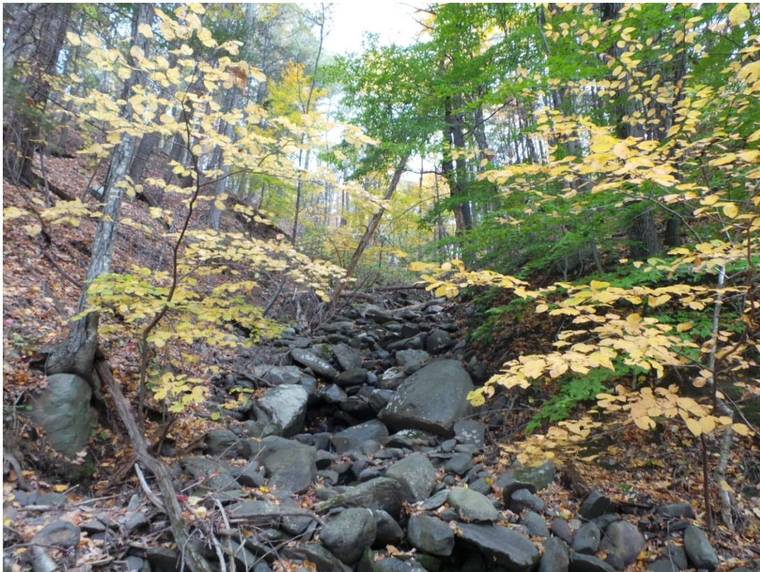
Photo 420 – Erosion of hillside draining down into blocked culverts
