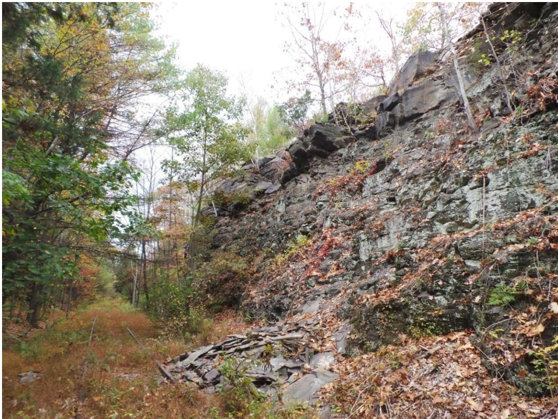
Photo 108 – Rock slide (station rr 550+00)
