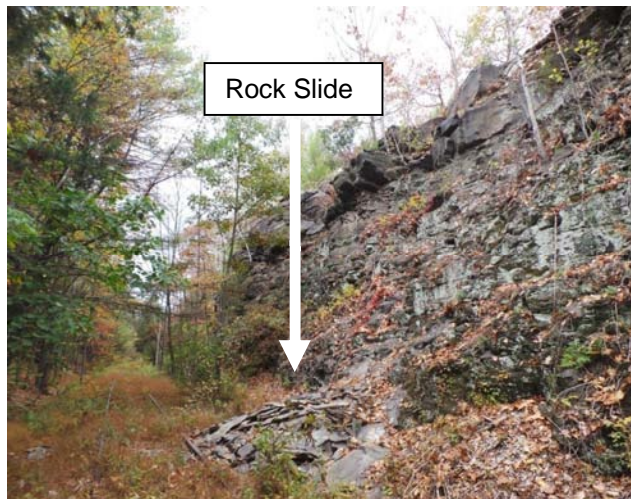
Photo 1-5 Rock Slide in Segment 1
