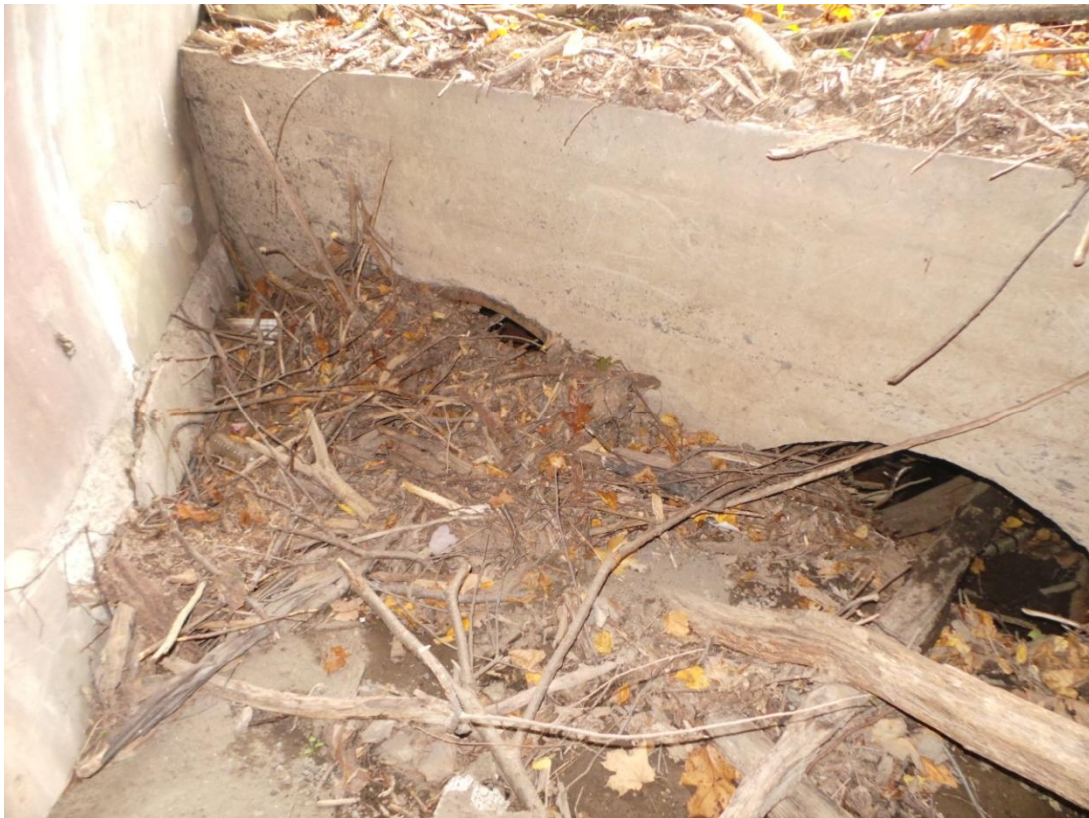
Photo 418 – Two 48” diameter steel culverts nearly 100% blocked with debris
