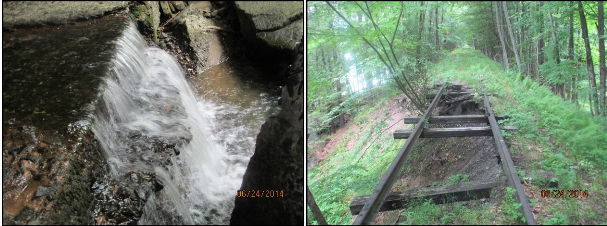
Scour at DS End of Culvert
