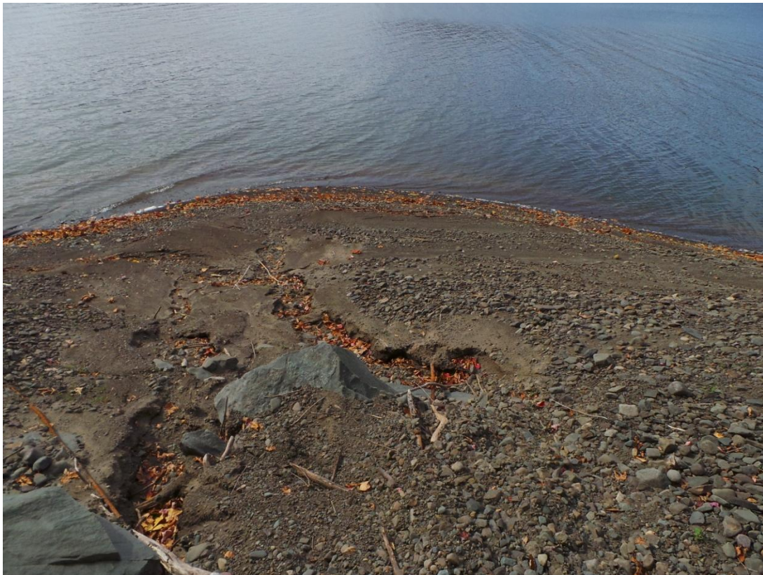
Photo 422 – Erosion and sediment deposition on the Ashokan Reservoir shore
