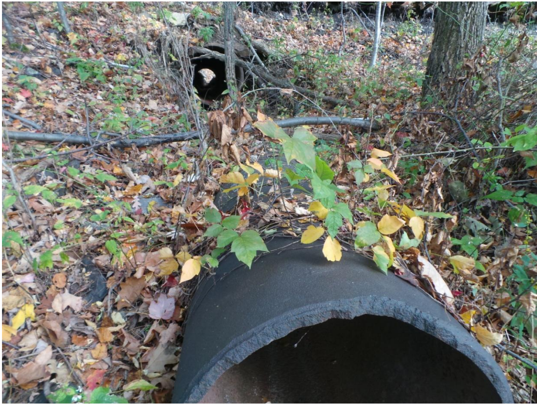
Photo 415 – Complete separation of a section of drainage pipe
