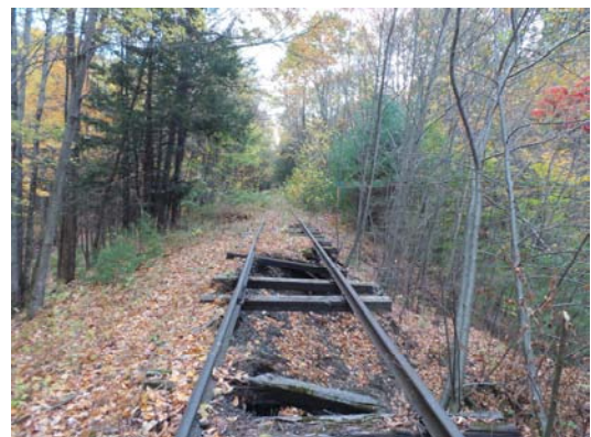
Photo 3-1 - Severe Deterioration in Segment 3
