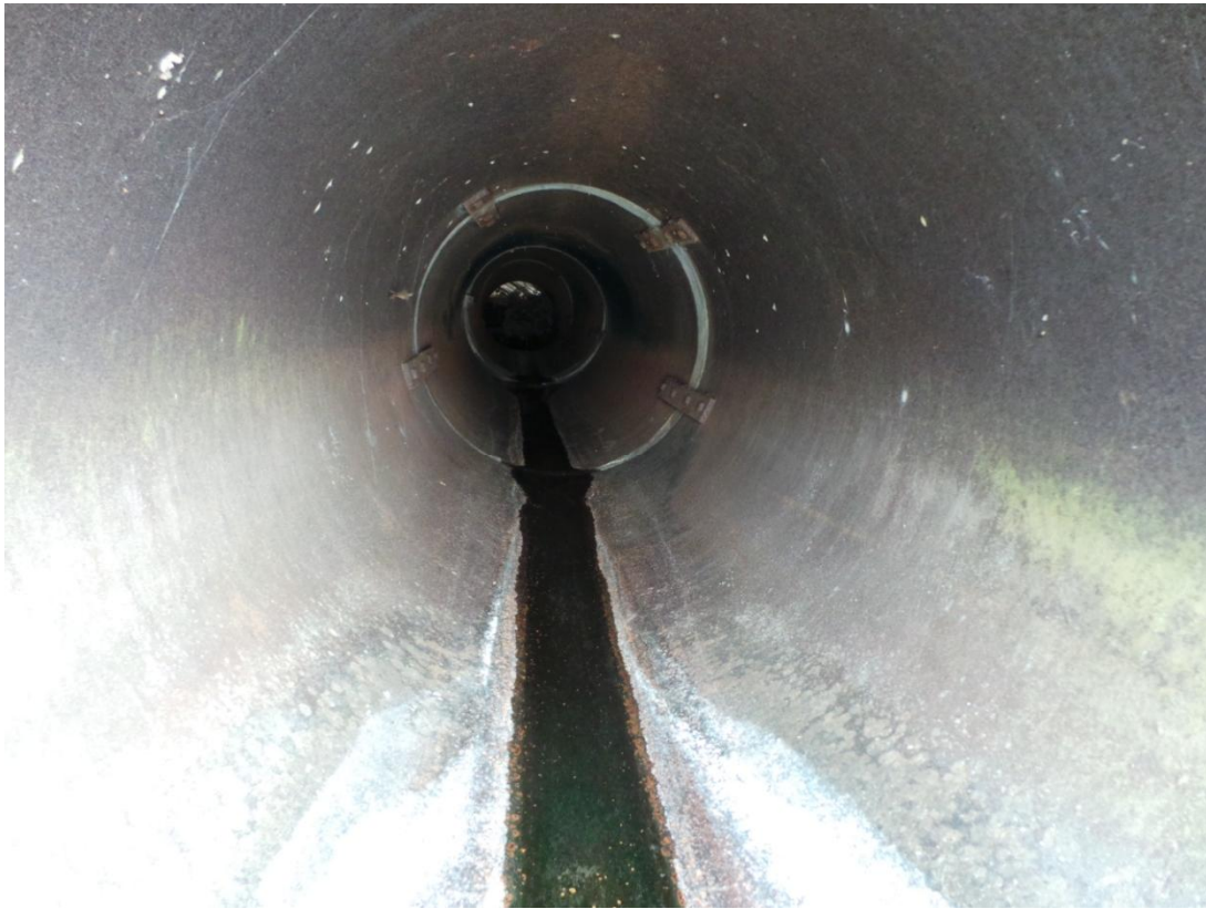
Photo 417 – 48” diameter steel culvert showing greater than 75% blockage
