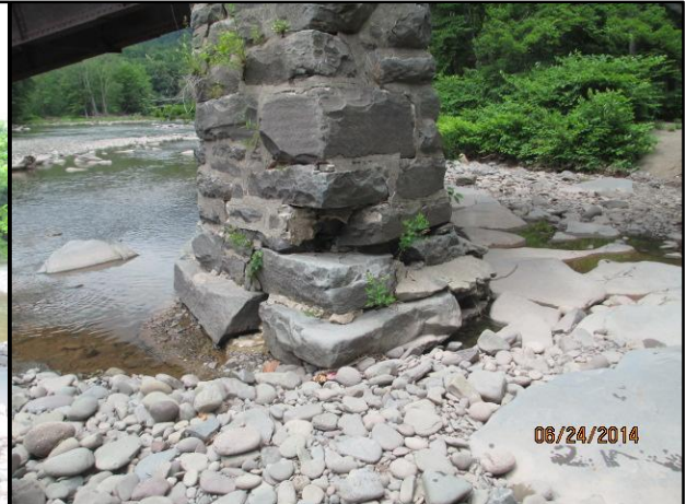
Pier 1 – Scour/Dislodged Stones
