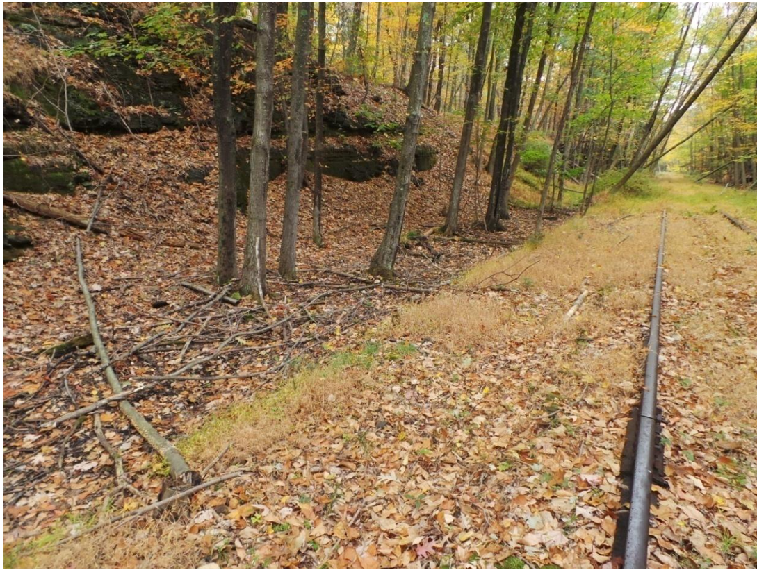
Photo 113 – Drainage Ditch requiring tree/debris removal
