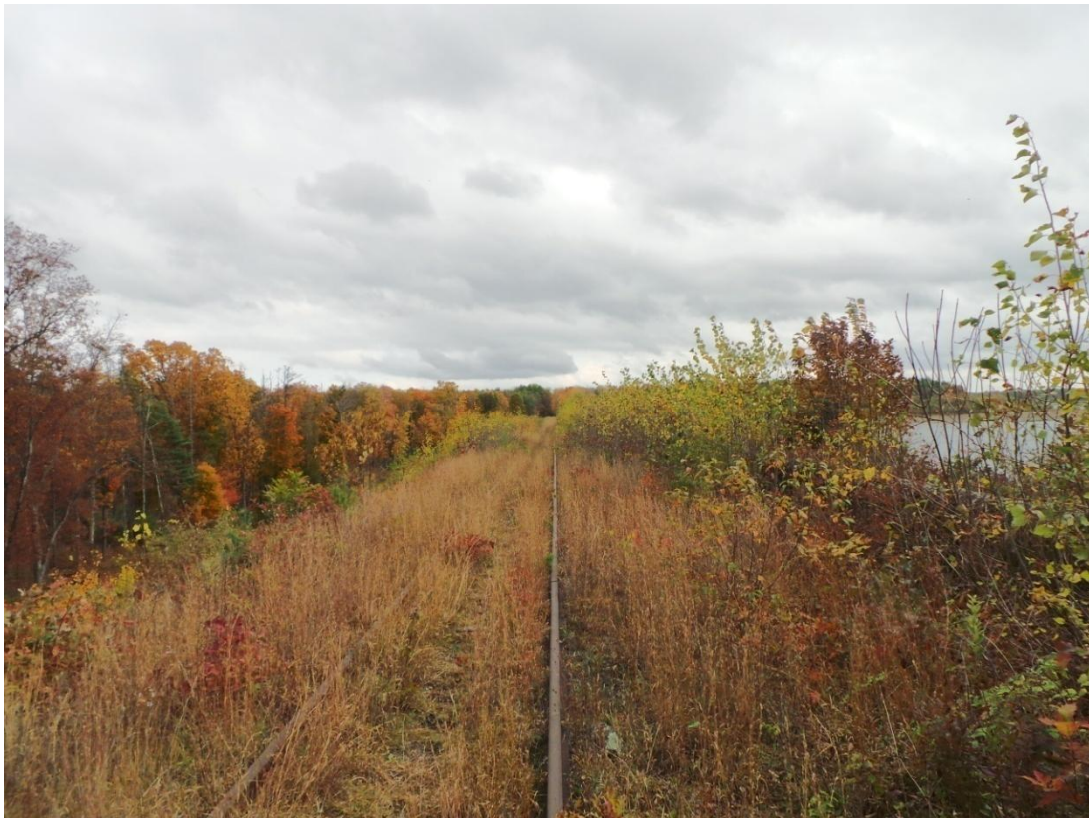
Photo 104 – Vegetation growth at the top of the Glenford Dike
