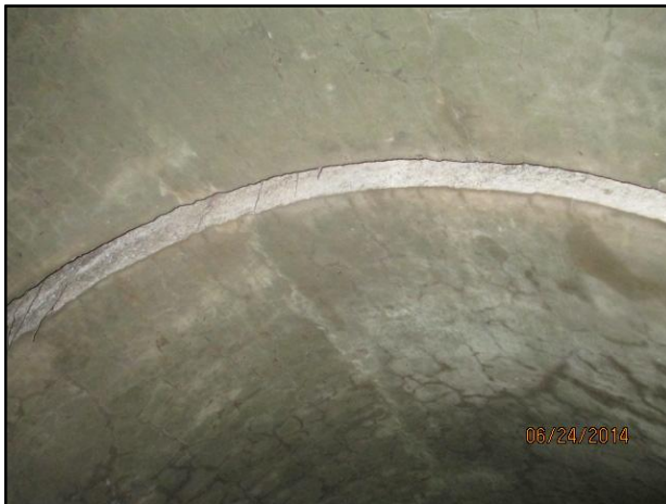
Crack in Culvert Barrel
