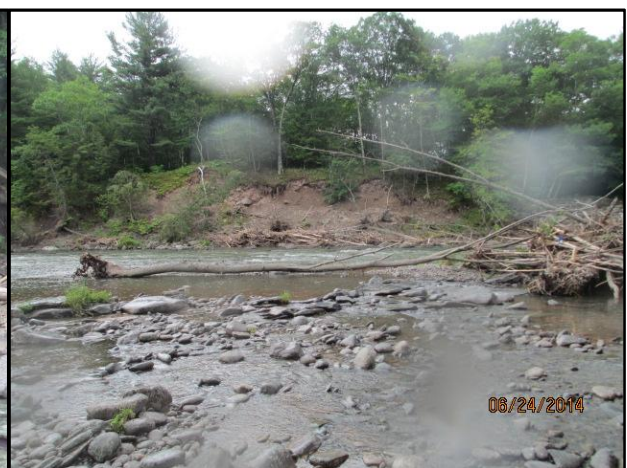
South Stream Bank Erosion
