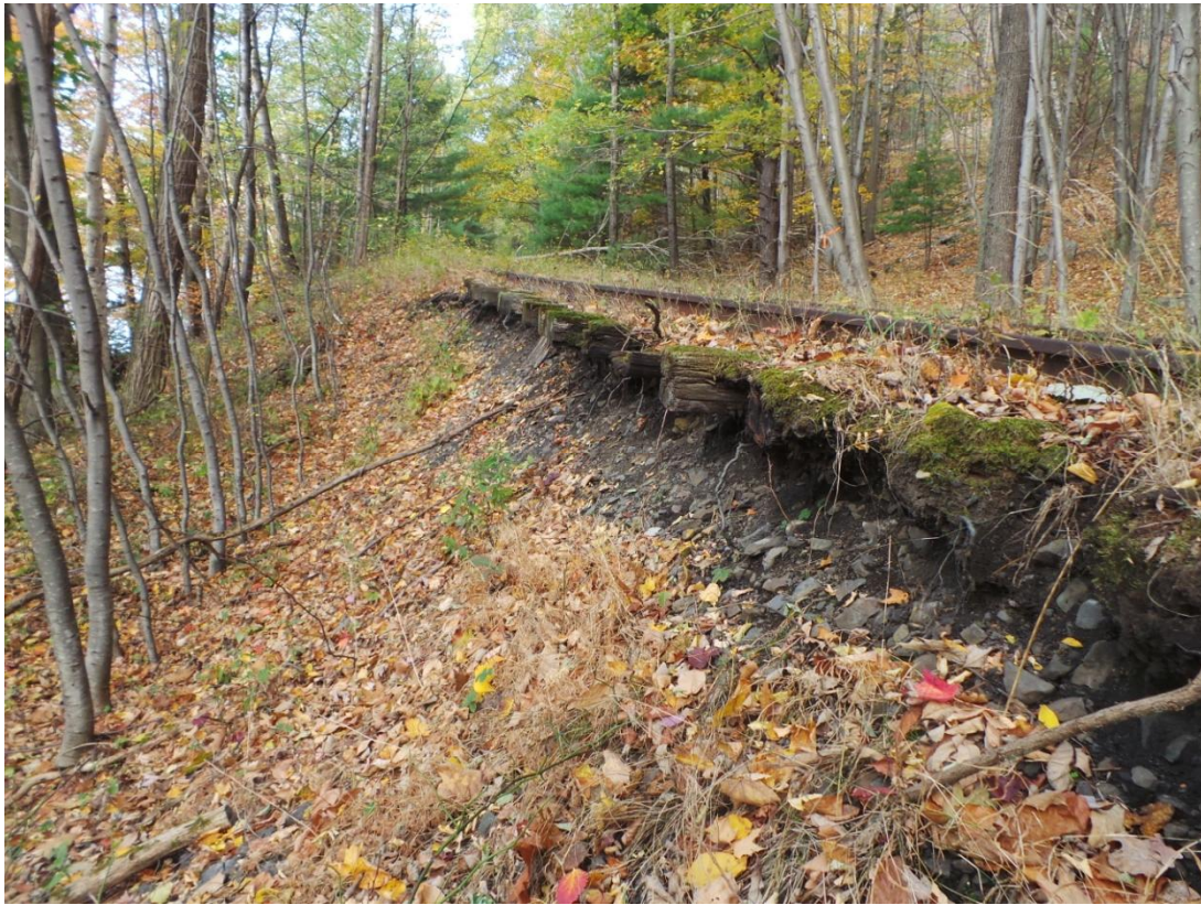
Photo 413 – Erosion of ballast and embankment
