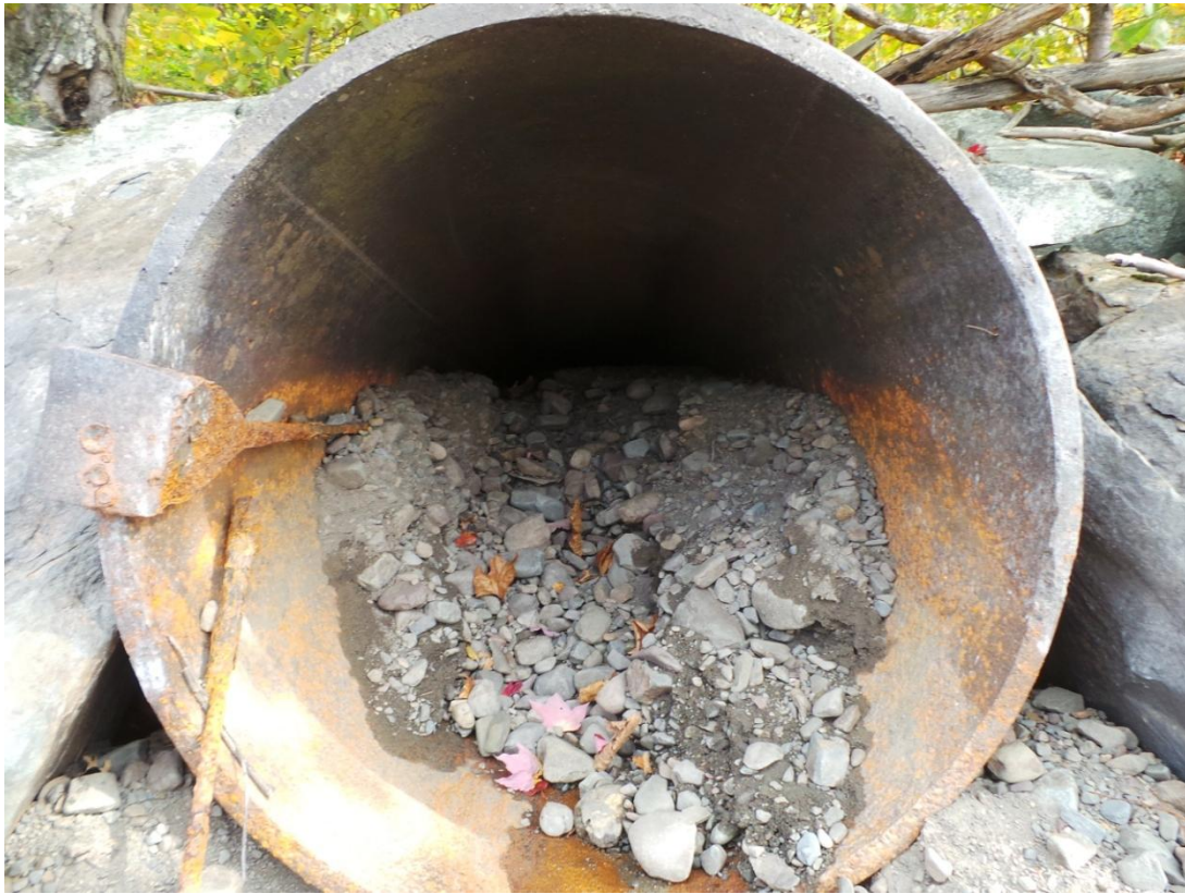
Photo 421 – Stone and sediment blockage at outlet of steel culvert
