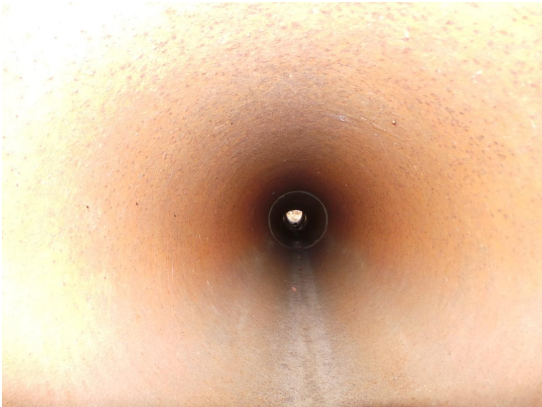
Photo 416 – Settlement/sag of steel culvert
