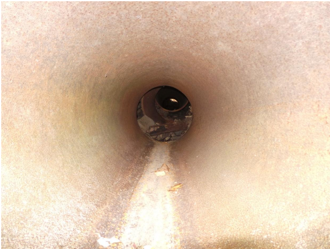
Photo 424 – Separation of three different culvert sections
