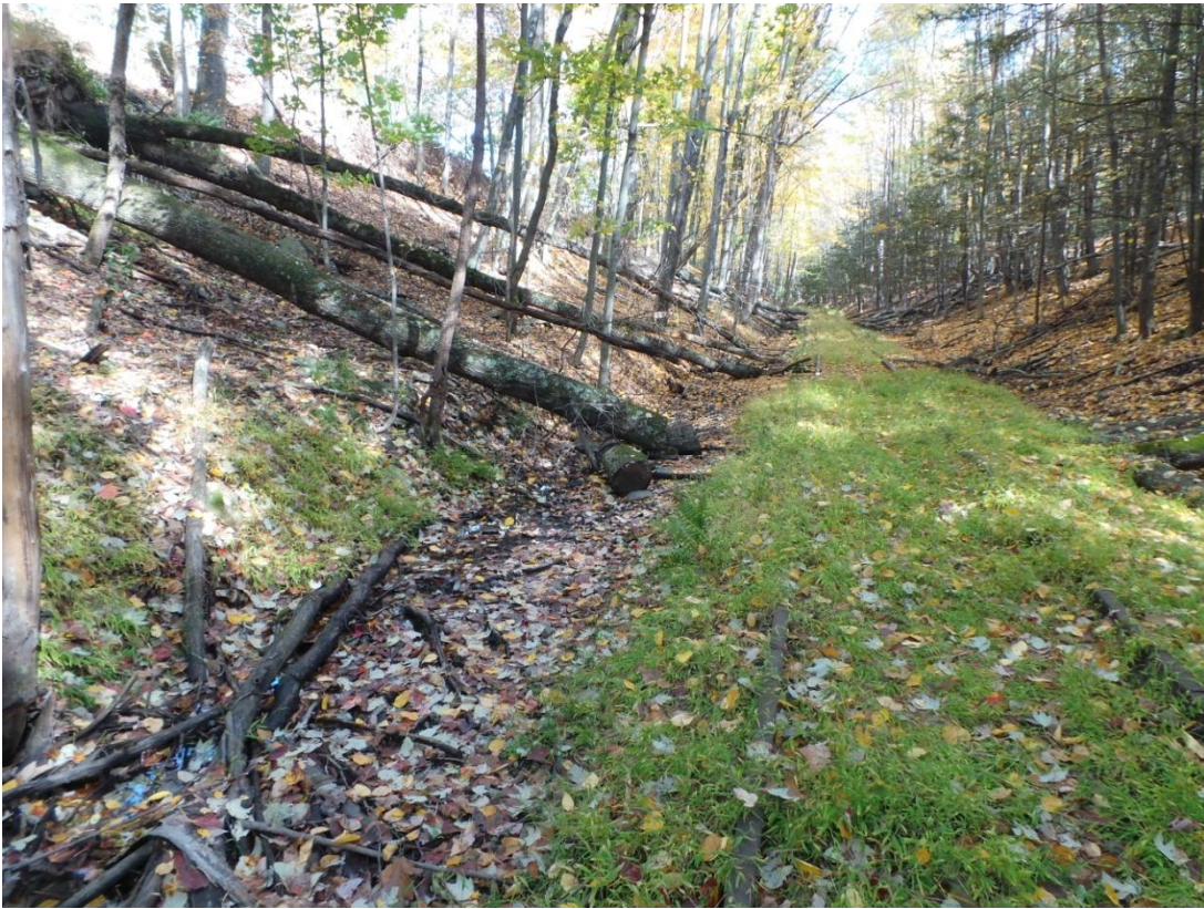
Photo 209 – Drainage ditch with significant debris accumulation
